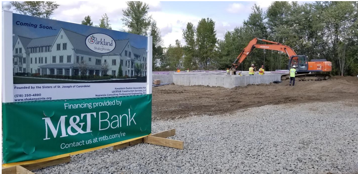
Work begins at the site of Shaker Pointe's new building, Parkland at Shaker Pointe, which will offer rental opportunities for residents.
